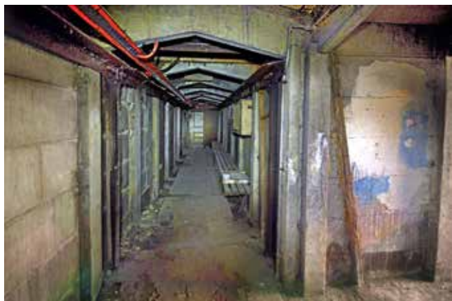
Benches still in place in the Grainger Market shelter. Note the wooden framework for a gas curtain on the right.
